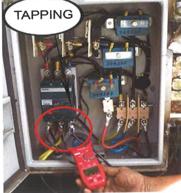
UNAUTHORISED TAPPING FROM K.M.C. KIOSK AT B.K.ROAD. EKBALPORE P.S.
