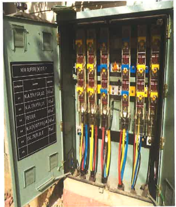
Modified Pillar box
