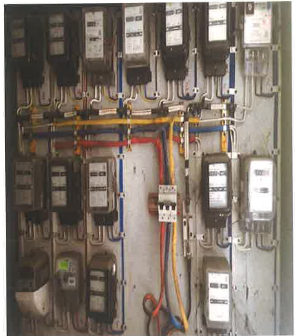
MCB replacing conventional cut-out
