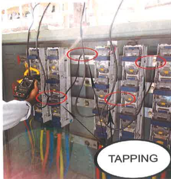
UNAUTHORISED TAPPING FROM PILLER BOX AT TOPSIA 2ND.LANE. TILJALA P.S.
